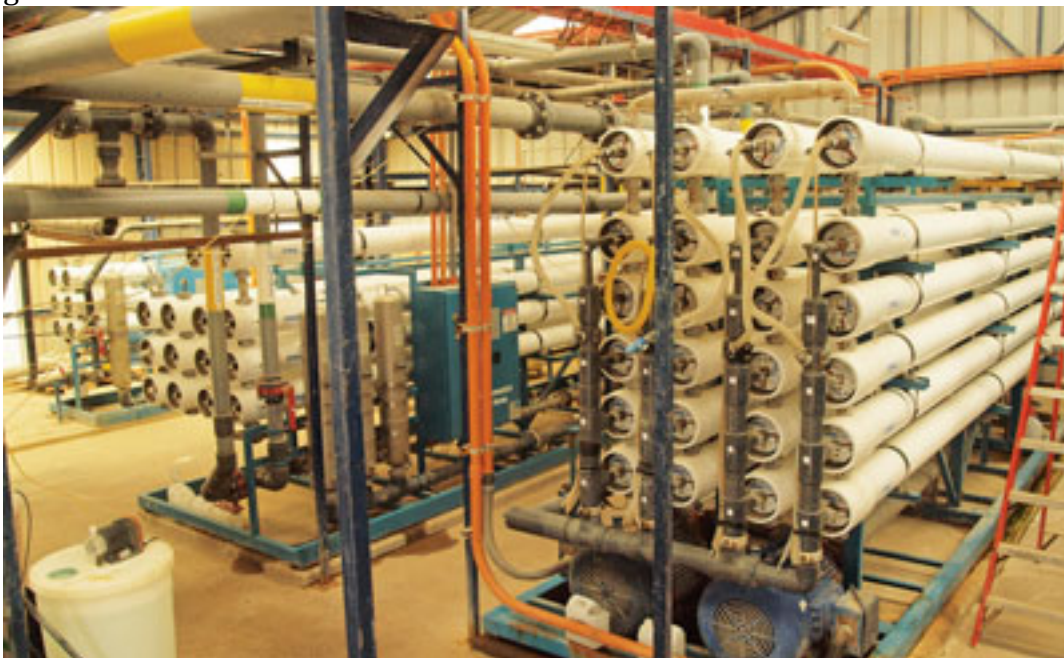
Under scrutiny: new reverse osmosis facilities coming online in Chile will be subject to tough environmental and quality standards
